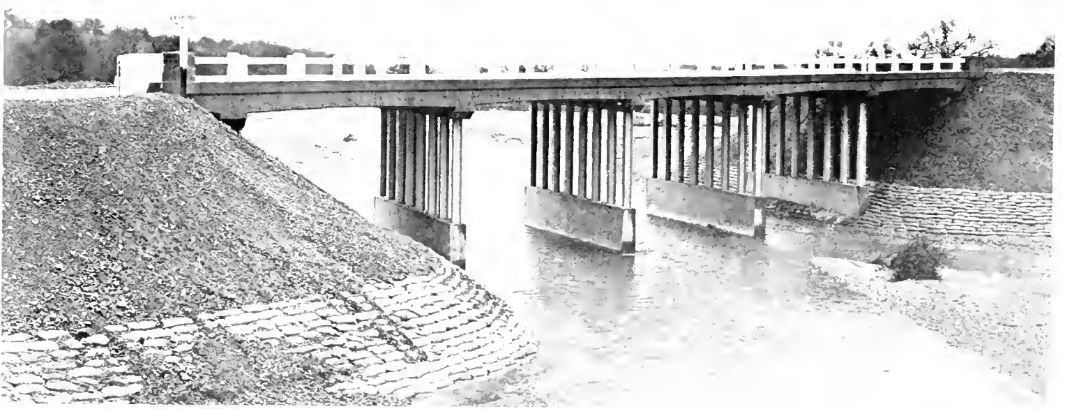
Six mile relocation of U. S. 99 north of Red Bluff just completed includes a 160-foot concrete slab bridge on steel piles across Dibble Creek and a 135-foot bridge of same type across Blue Tent Creek shown in top and bottom photos
